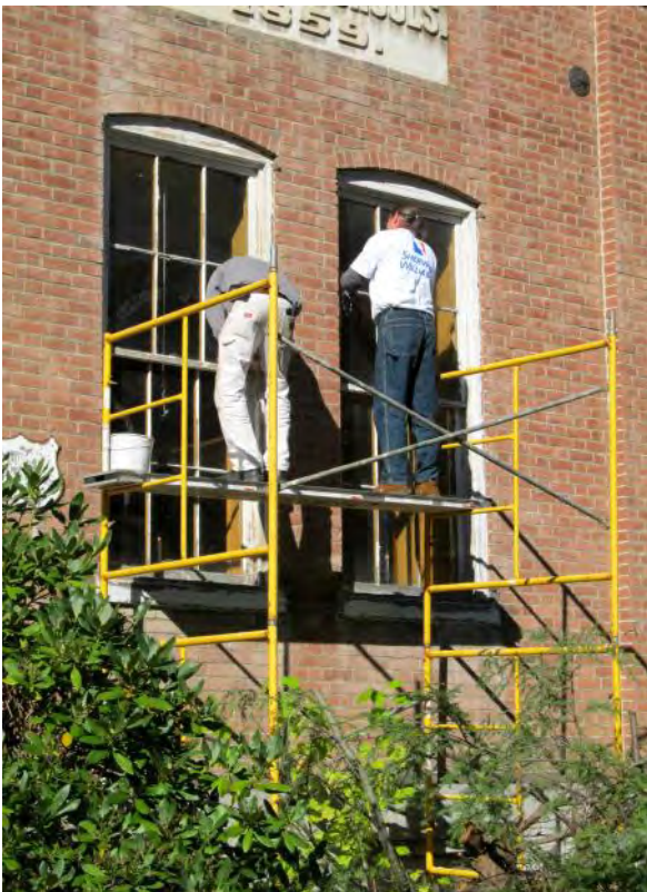
Painters preparing Surfaces of Windows and Window Frames in East Wall for Painting
