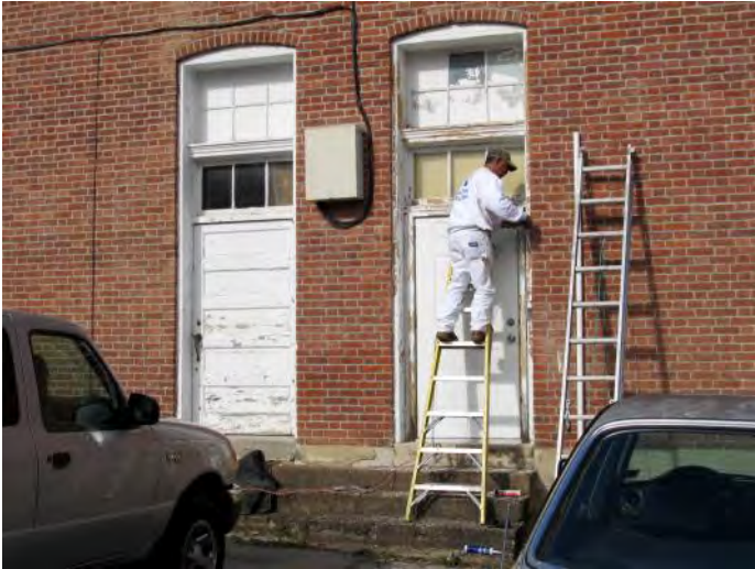
Painters preparing Surfaces of First Floor Doors and Transoms in South Wall for Painting
