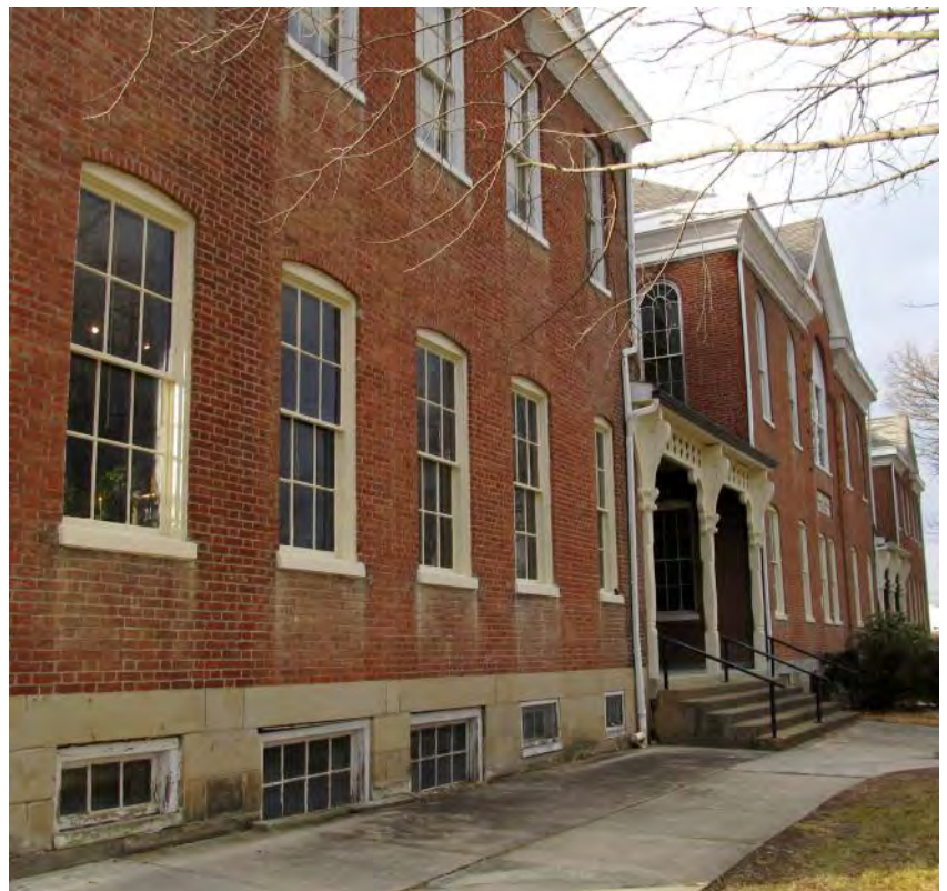
Painting of the First Floor Windows and Porch Trim in East Wall Completed
