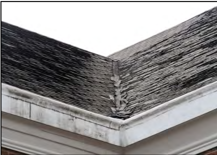
Museum Roof Section in Need of Repair
